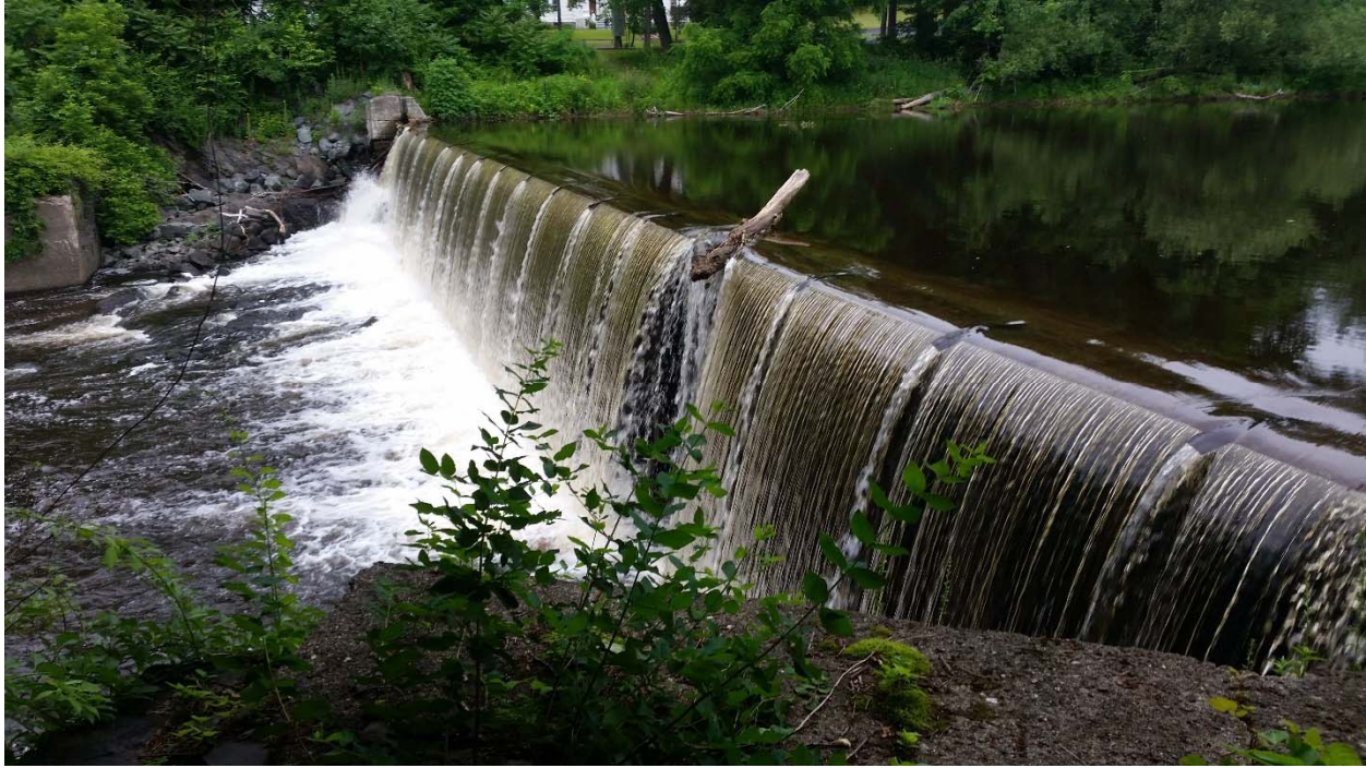
Figure 11. Mt. Ida Dam, located on the Poesten Kill in Troy, NY. (Photo credit: OEI)
